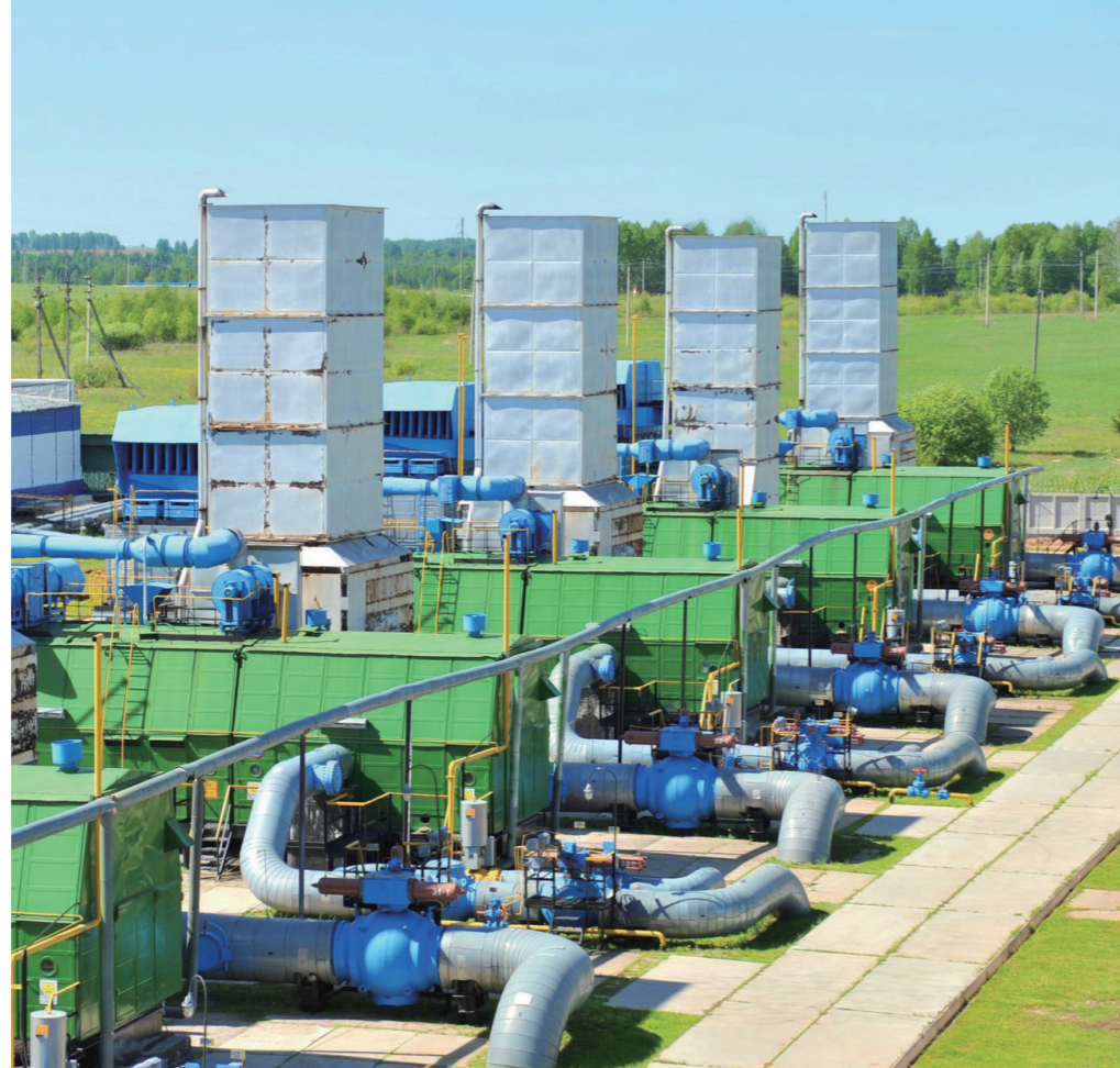
Natural Gas Pipeline Compressor Stations
